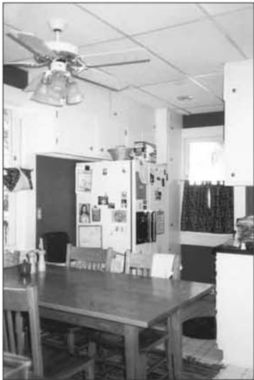
Before Provided by Farstad family The old kitchen had a suspended ceiling and little room for the appliances and dining table.
